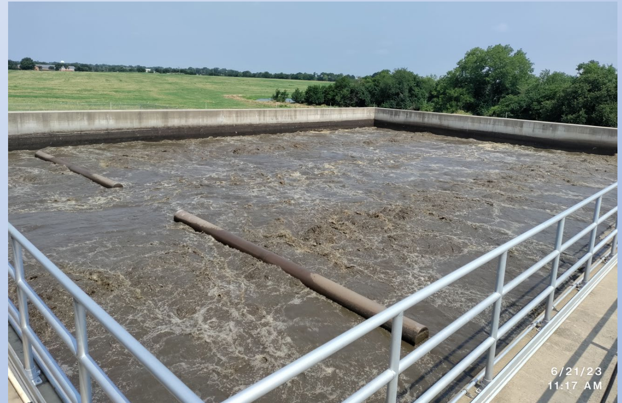
Sequencing Batch Reactor Tank #1 in React Mode
