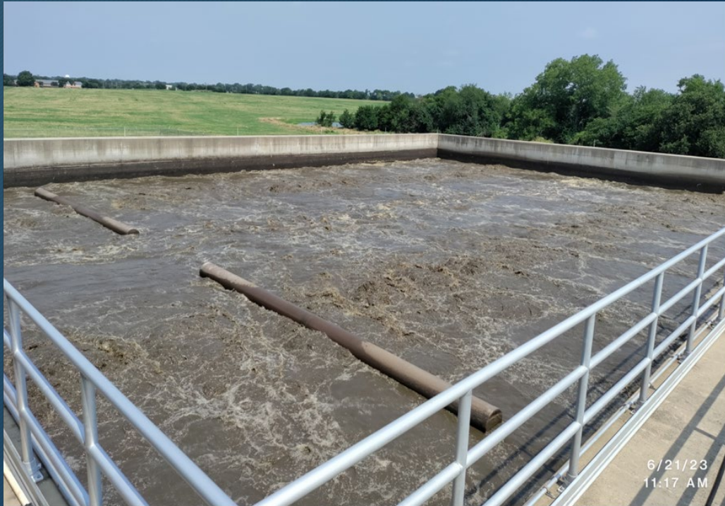
Sequencing Batch Reactor Tank #1 in React Mode
